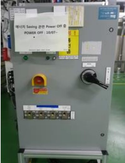
PUMP Power Rack
